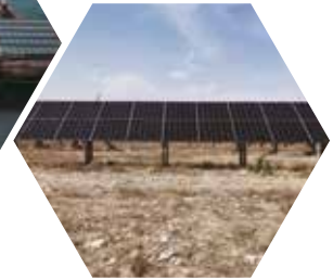
Ground-mounted Photovoltaic Power Station, Yinchuan
